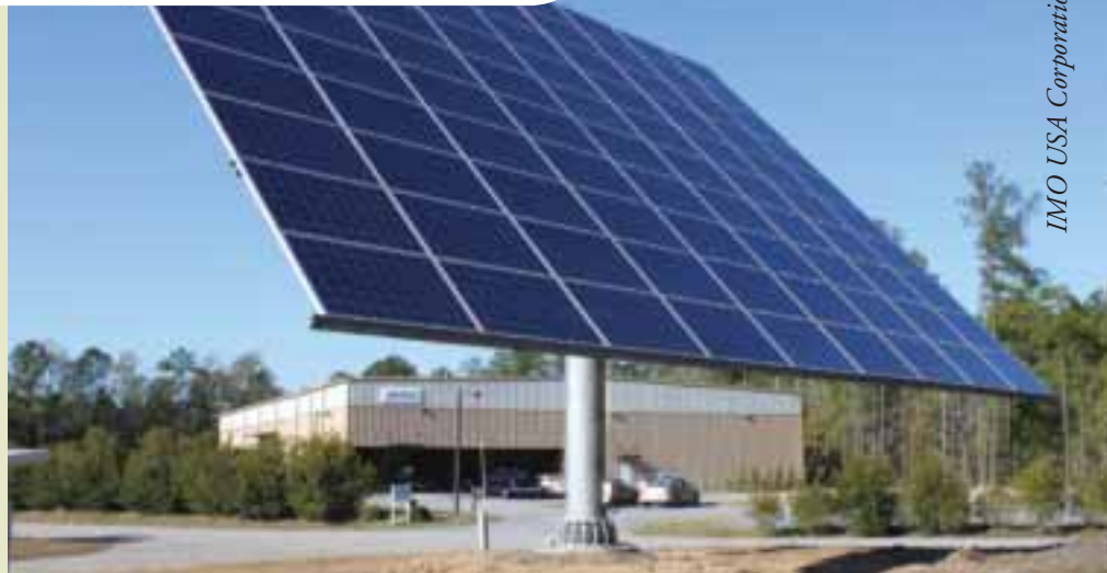
Solar Tracker – IMO USA has built and installed a giant “Solar Tracker” next to its plant in Summerville, S.C. The Solar Tracker powers 40% of the factory's building operations (excluding production machinery) by rotating to face the sun's brightest spot and then pumping electricity into the adjacent warehouse.
